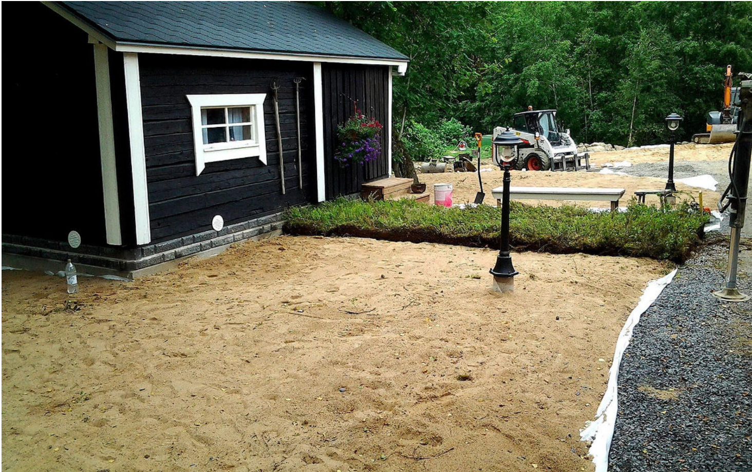
Example of groundwork: A landscape fabric has been spread over the area reserved for forest mat, and it has been covered with an approximately 10 cm layer of fine sand.
